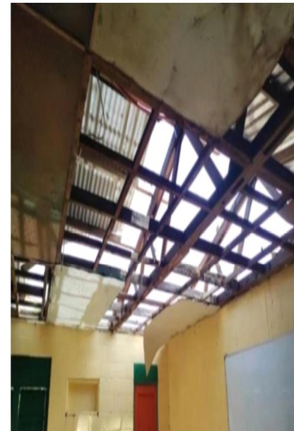
Onesua College - Damage to Junior Science Lab
