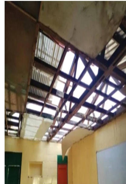
Onesua College - Damage to Junior Science Lab
